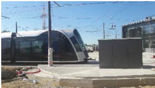
Caption image 2: Compact control cabinets can replace oversized technical rooms and can be handily integrated into the architecture at the stops and transfer platforms.
